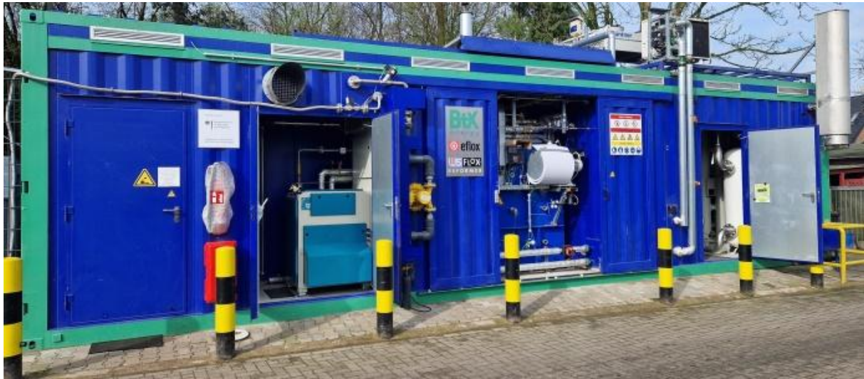
Figure 3: Demonstration plant for the production of 100 kg biogenic hydrogen / day
